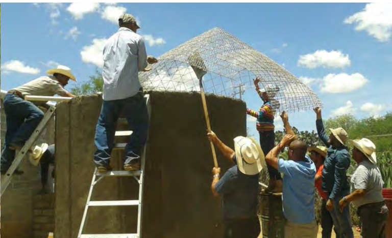
Local community residents come together with Caminos de Agua to build a much-needed rainwater harvesting system.
