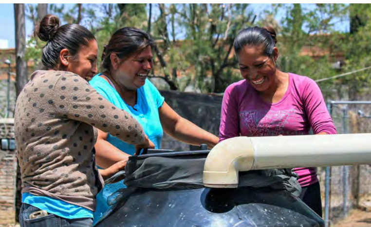
Local women assembling a component of a rainwater harvesting system on a Caminos de Agua project.
